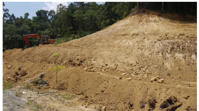
Constructing retaining wall by putting up gabions at Timimbang Base Camp to prevent the loose soil from sliding down
