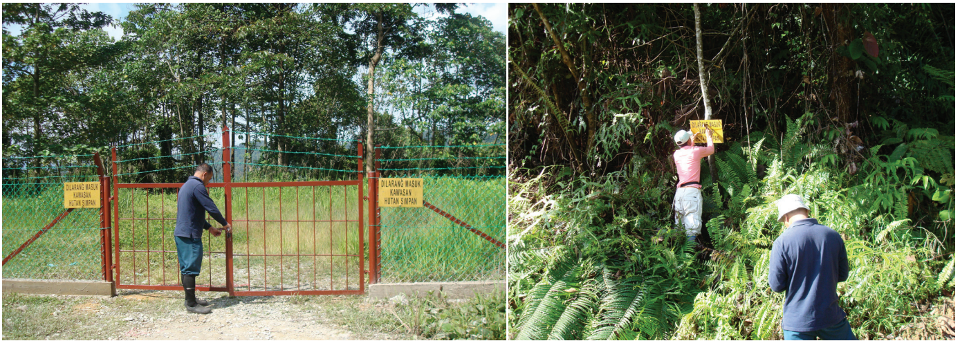
(left) Putting up fence at Compartment 10 and (right) fixing FD plates as a means to deter people from entering the forest.
