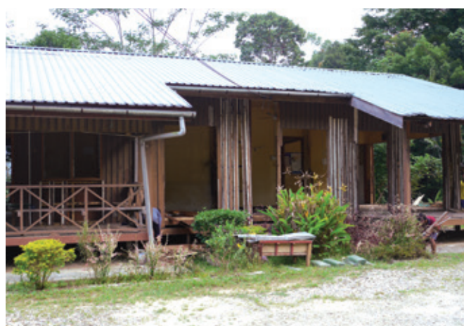
The staff quarters to be demolished due to termites infestation.
